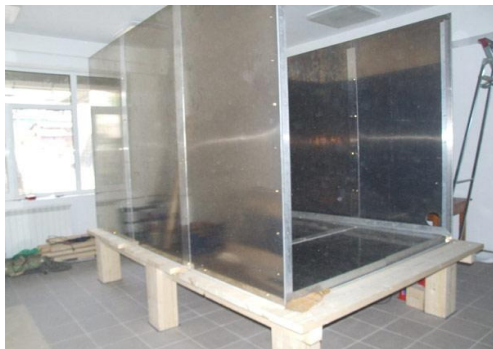
Fig. 1. Shielded room against the spurious microwave signals for radiometric operations, during the construction
